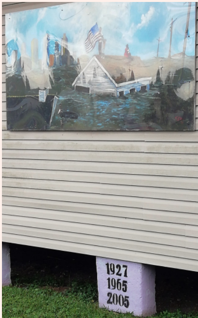
Fig. 2. A painting on the museum's exterior. The dates on the foundation refer to three different devastating floods.
